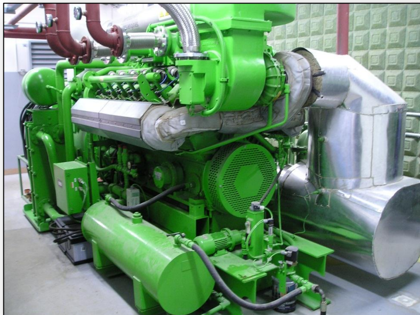
CHP unit - 625 kW e
