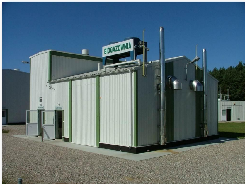
Technical building with hygienizator and CHP unit
